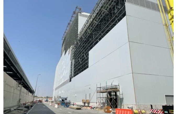
The final panels in the boiler hall west wall are being fitted
