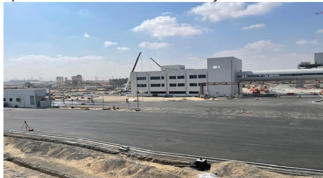
The main access road through the weighbridges onto the tipping floor is now completed
