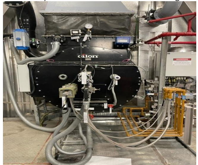
Oil burners inject diesel fuel into the combustion chamber at level 17 meters
